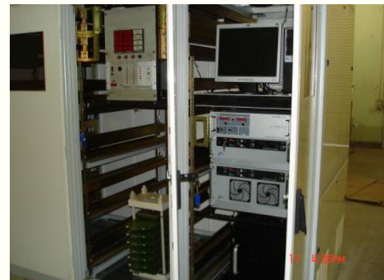
Power supplies integration
